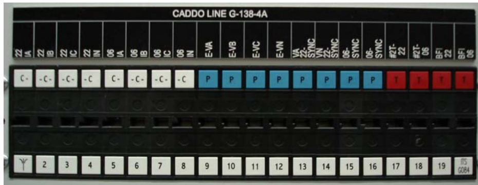
Figure 3. 20-Pole Test Block Used for a Line Distance (21B) Relay
