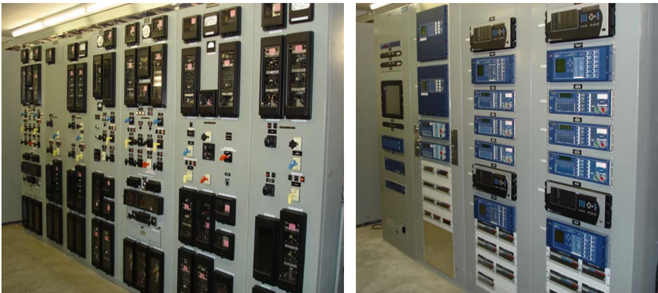
Figure 6. Retrofit of Relay Panels for a Breaker and a Half Configuration
