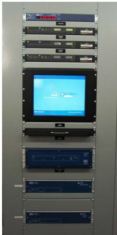
Figure 8. Substation HMI Panel Front View
