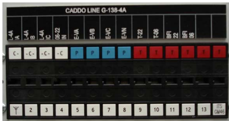
Figure 4. 14-Pole Test Block Used for a Line Differential (87L) Relay
